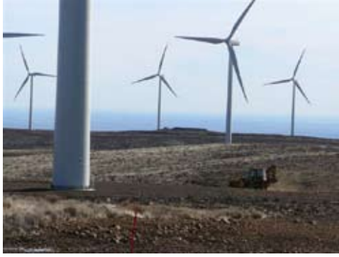
Morgan & Son Earthmoving doing road maintenance work at the Wild Horse Wind and Solar Facility near Ellensburg, WA.
